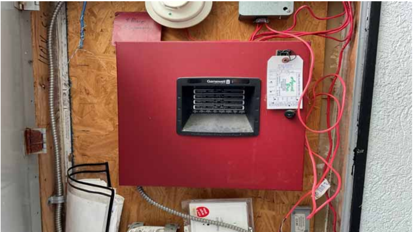
Fire Alarm Panel - Typical
