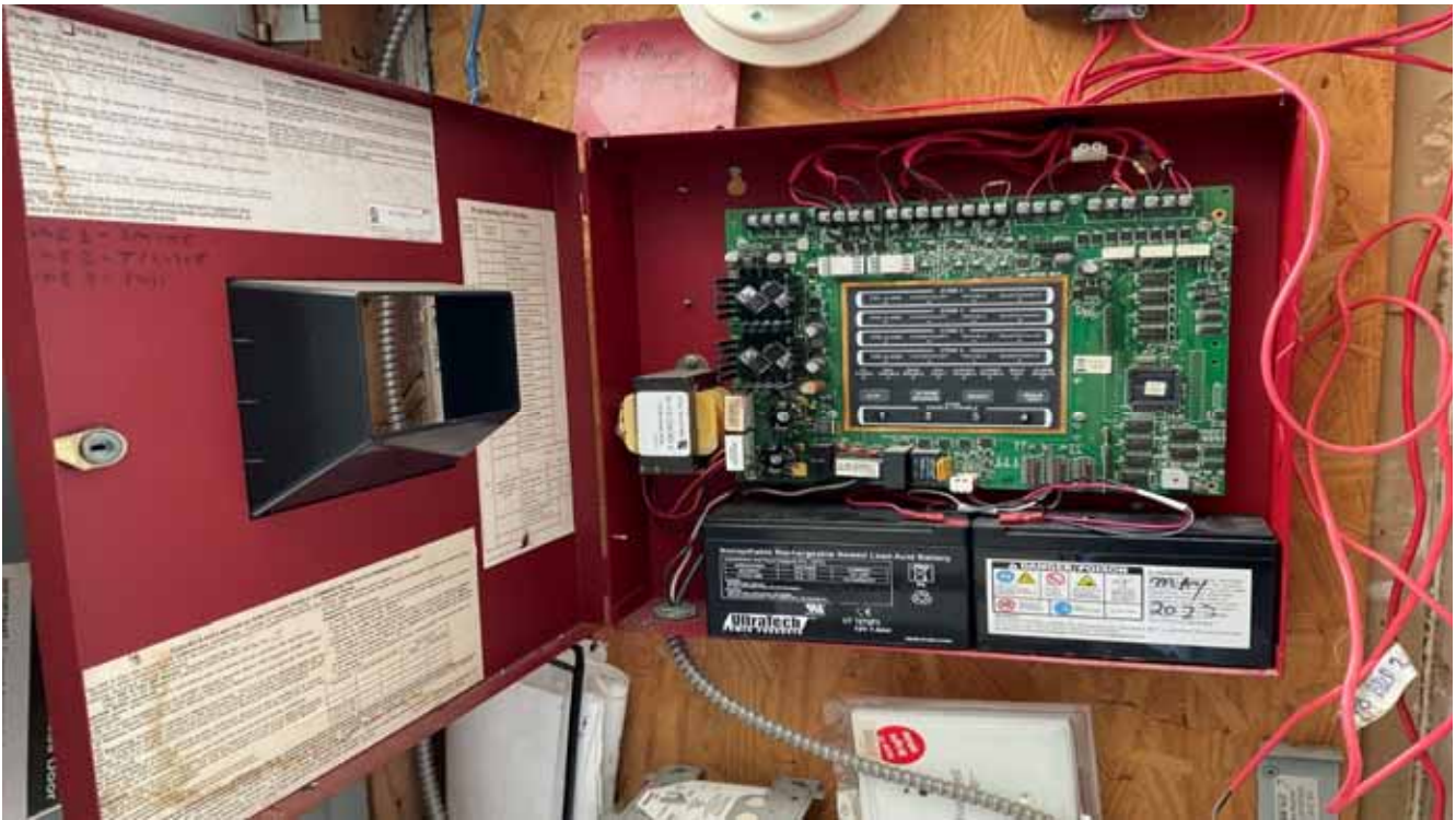
Fire Alarm Panel - Typical
