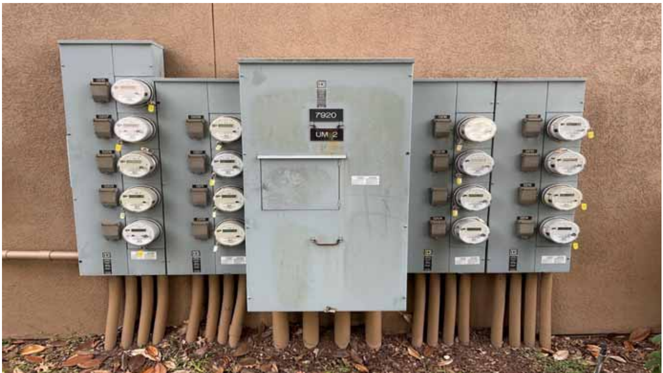
Electrical Meters - Typical
